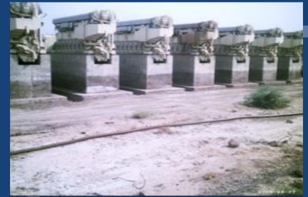
CLIENT: IRAQI MINISTRY OF ELECTRICITY
