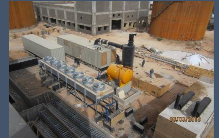
CONTAINERIZED GENSET CONFIGURATION
