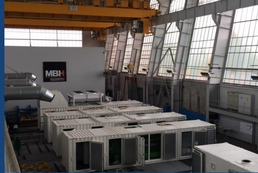
7 CONTAINERIZED GEN-SETS POWERED BY JENBACHER GAS ENGINES AND ASSEMBLED AT MBH FACTORY IN GERMANY
