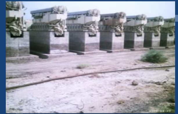
CLIENT: IRAQI MINISTRY OF ELECTRICITY
